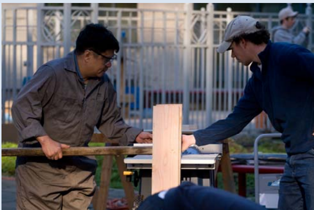
Downtown YWCA: UBC students researched structural designs and appropriate layouts, then constructed a rooftop trellis system to grow vines (such as raspberries)
